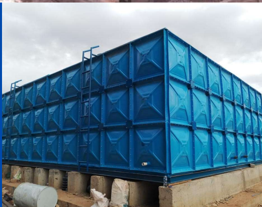
Water Storage Tank
