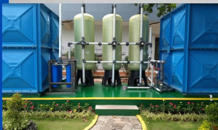
SAND - FILTER - MANGANESE
