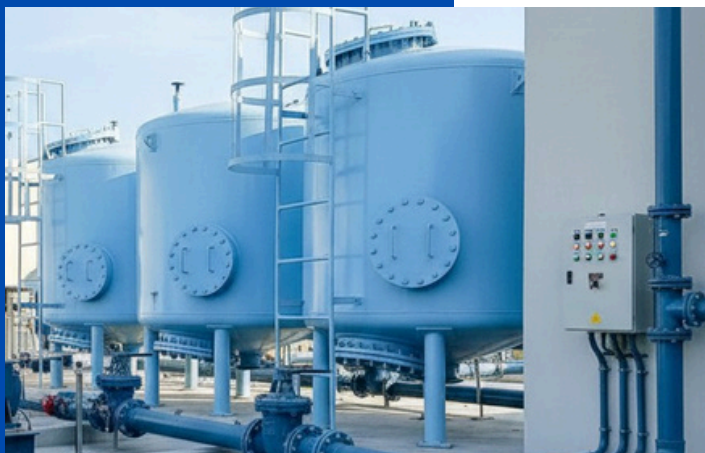
SAND FILTER & CARBON FILTER
