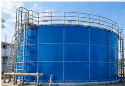
Fire Water Tank | Industrial Facility
