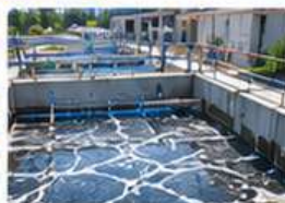
WWTP / IPAL Wastewater Treatment Plant
